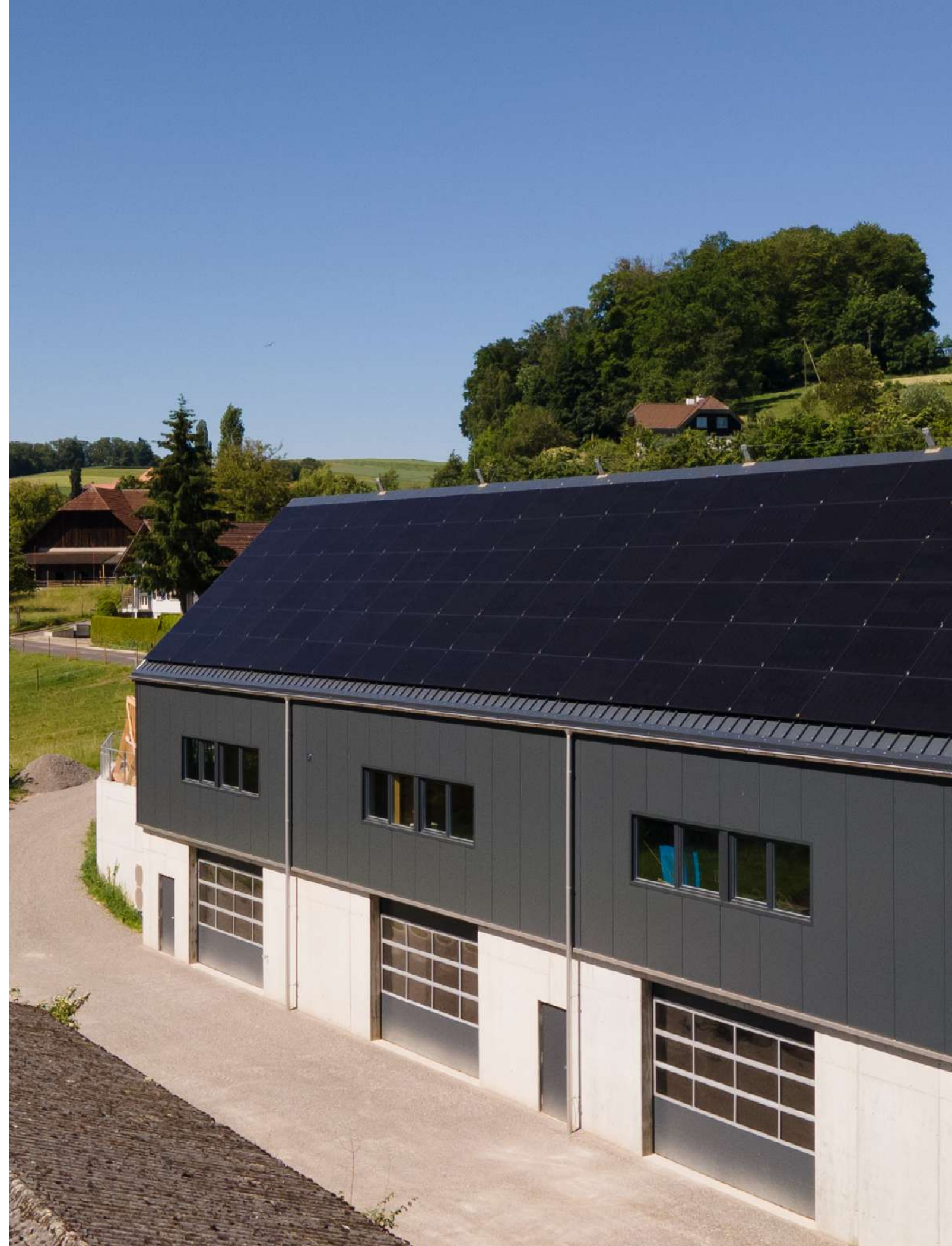
▲ Commercial hall in Buchegg | LOCKUP Roof | 182 m 2 | 36 kWp
