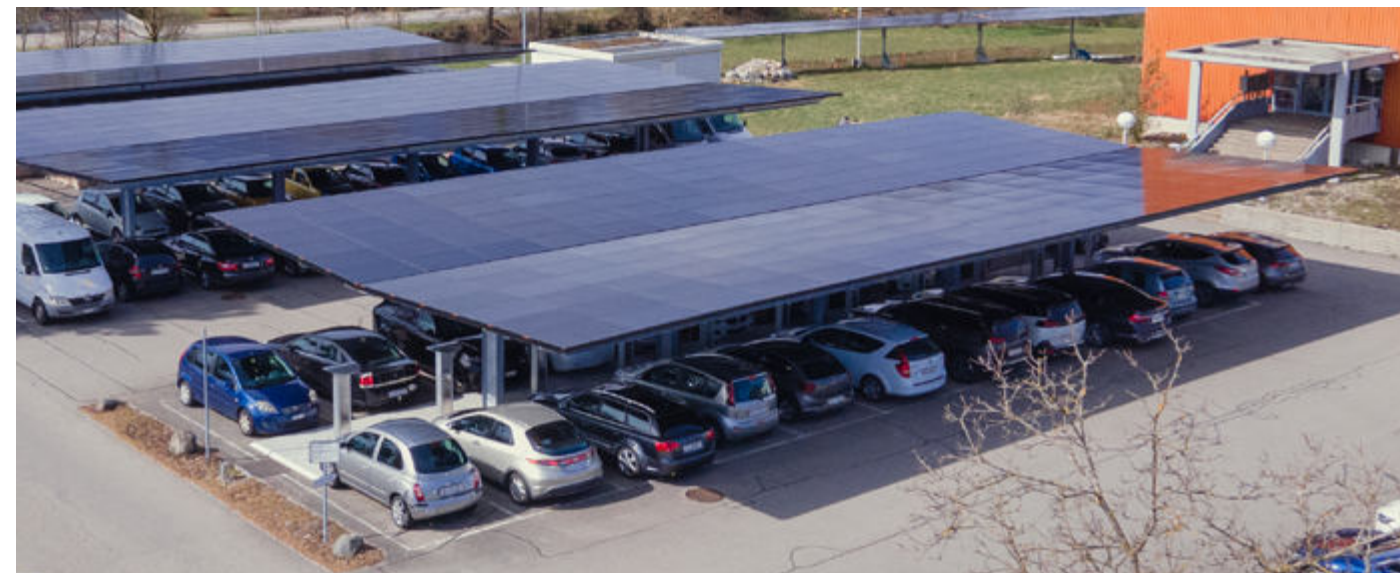
▲ Carport in Deitingen | Plant capacity: 222 kWp
